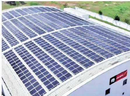
▲ Vietnam Plant / Solar panels
