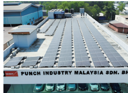
▲ Malaysia Plant / Solar panels
